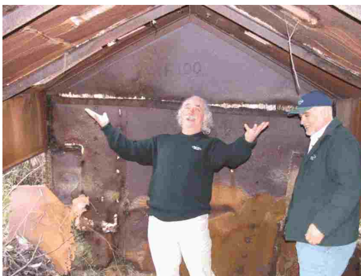
Ian Sullivan, Parks Victoria Heritage Coordinator and Ralph Angelico, Parks Victoria Gembrook Friends of Kurth Kiln Liaison Officer inspecting the Tonimbuk Kiln Structure.
